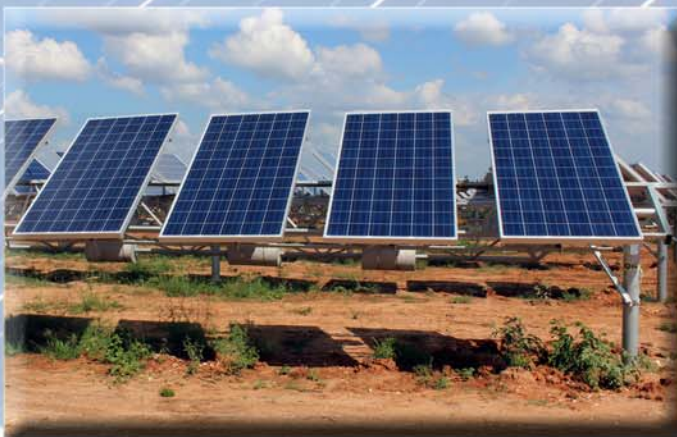
Dual-Axis SolarTracker Alamo 1 Project San Antonio, TX
